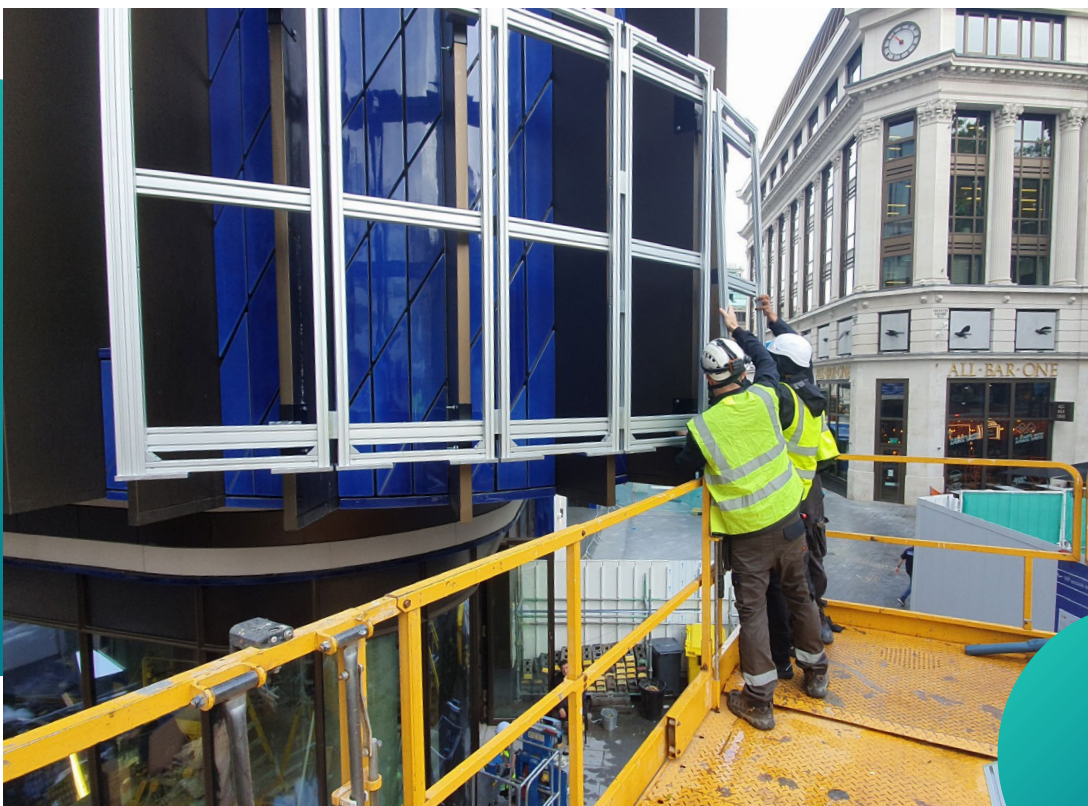
^ Installation of a bespoke framework onto a building with architectural fins within a severely restricted space
